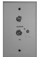
Antenna Power Supply
