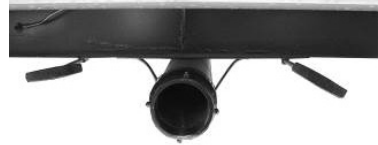
Black/Grey Tank Drain and Valves
