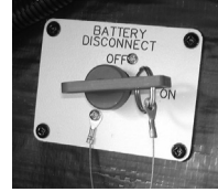
Battery Disconnect Switches
